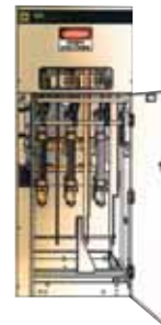
Interior view of disconnect switch and fuse assembly
