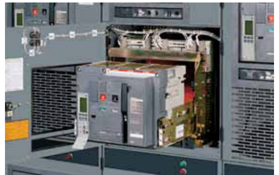
Masterpact NT breaker in its fully withdrawn position
